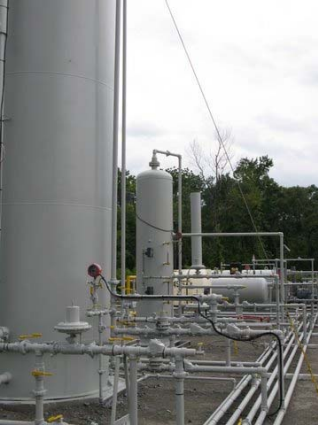
Two and Three Phase separators plus Heater treater for Jumonville # 1
