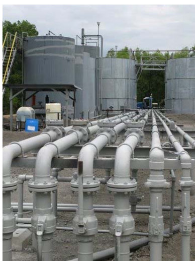
Tank Battery and Flow lines
